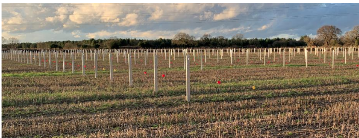
Figure 15.11-12 Mounting Structure Piles being Installed (taken at Tilm Farm, Retford, in January 2023)
