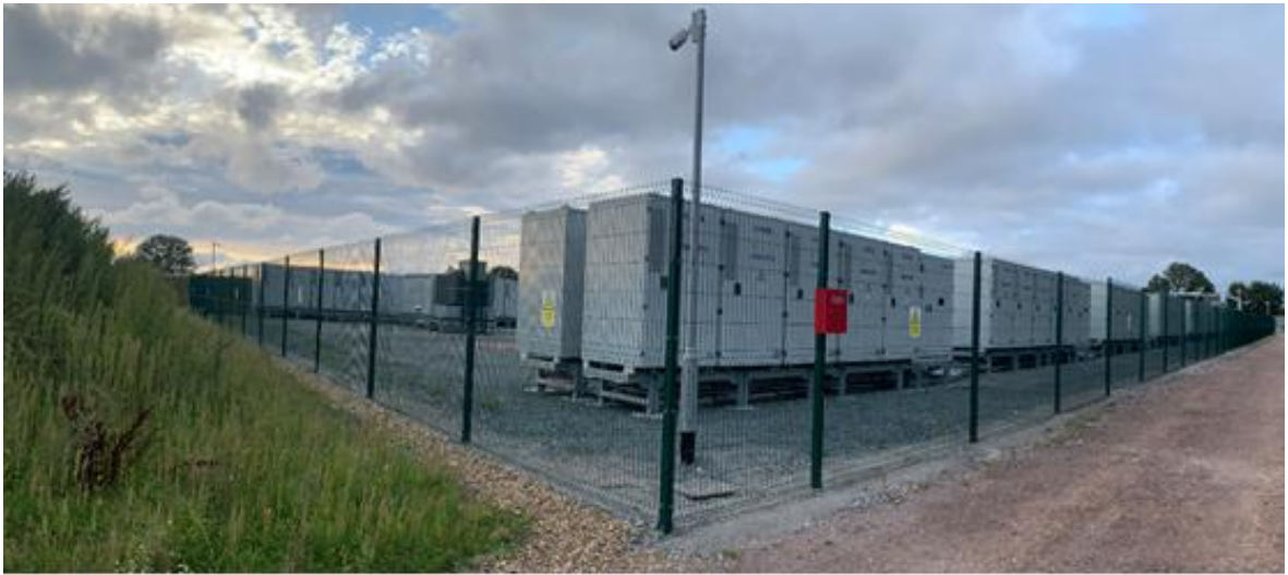
Figure 15.18-19 Example of a BESS
